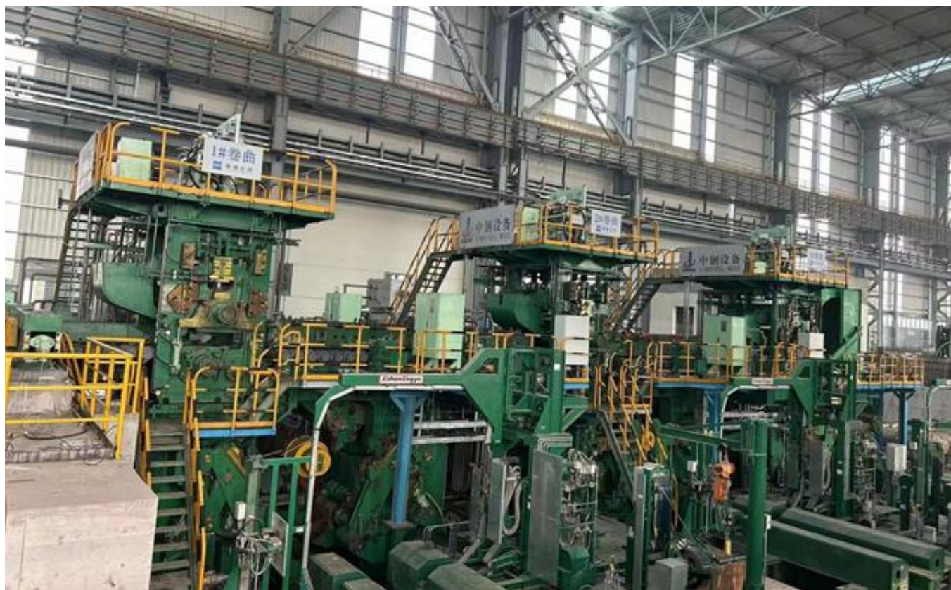
850热连轧机组 850mm Hot continuous rolling unit
